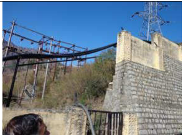
Connecting bay area for Nirmand Kotla line (outside the wall)
