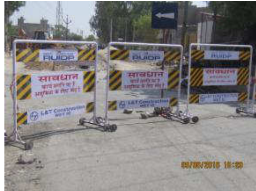
Caution and signage displayed at site
