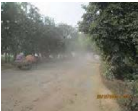
Broken pavement and dust emission at km 22.000
