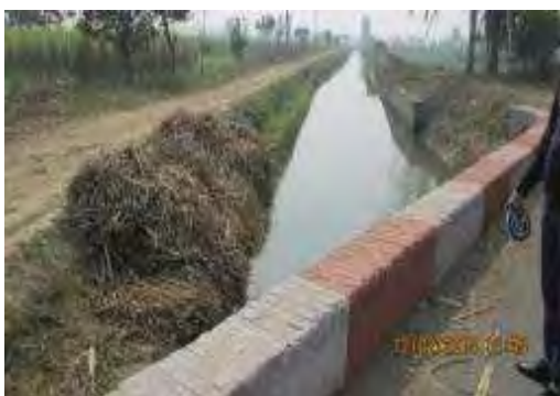
Fig.44: Canal at km 11.15 in Tawli
