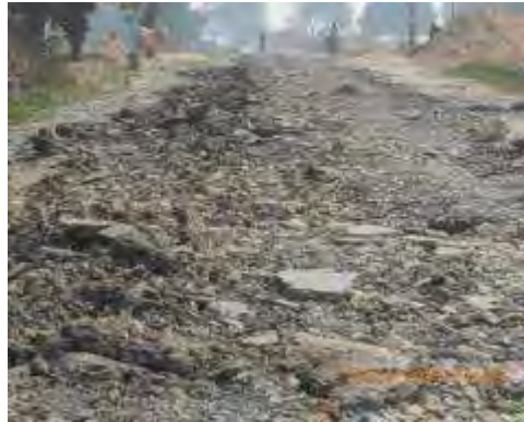
Fig. 119: poor road condition from km 9 to km 11 along Hussainganj to Alipur Marg
