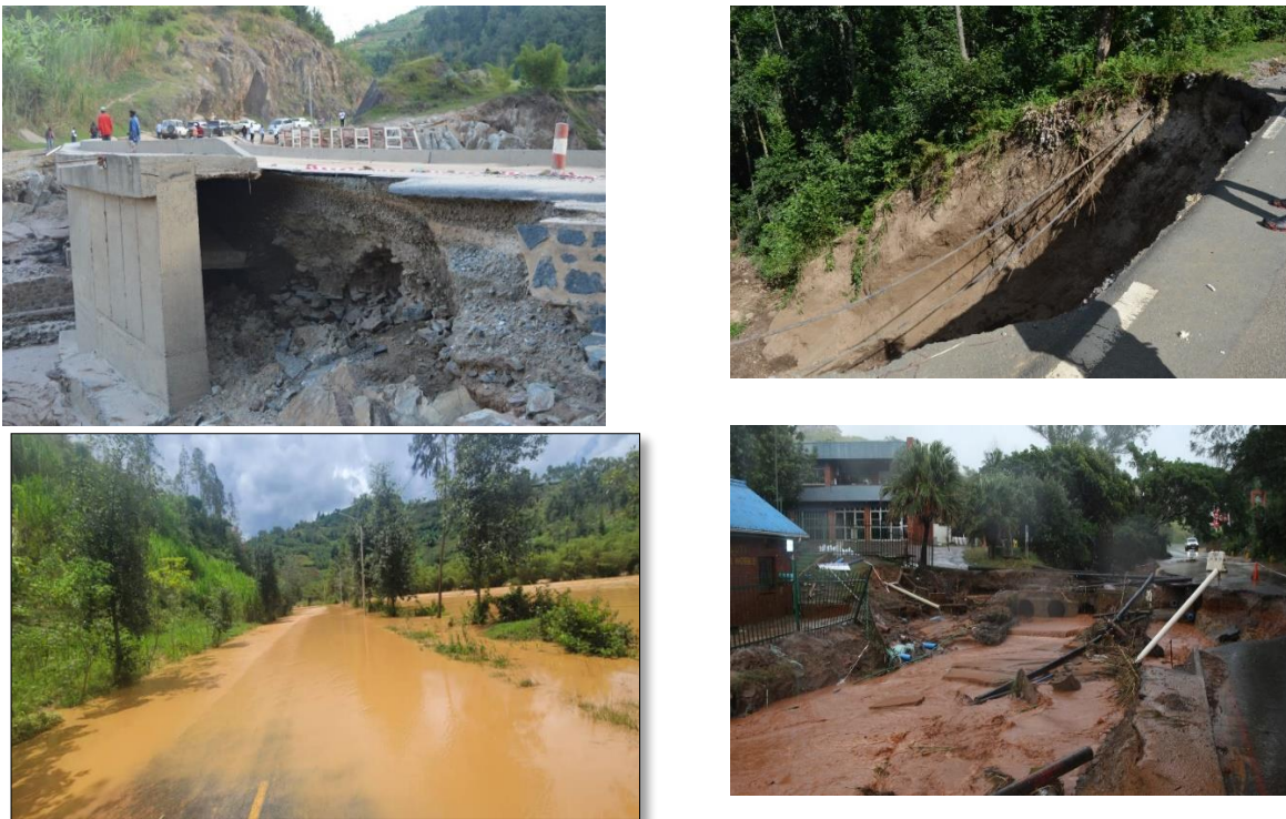
Figure 2: Typical features of floods affected project areas.
