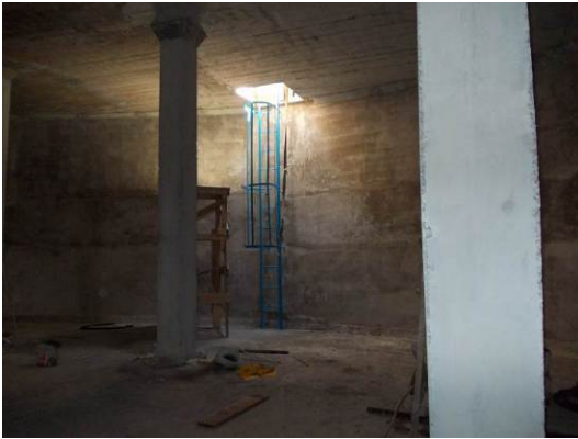
MES 01 – Wooden scaffolding used for plastering works – without protection
