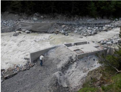
MES 01 – no sanitary fence upstream to Tyrolean weir (access unprotected)
