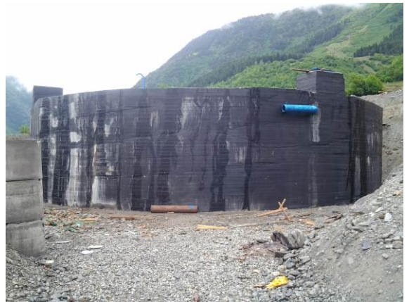
MES 01 – Backfill of reservoir pending leading to safety risks
