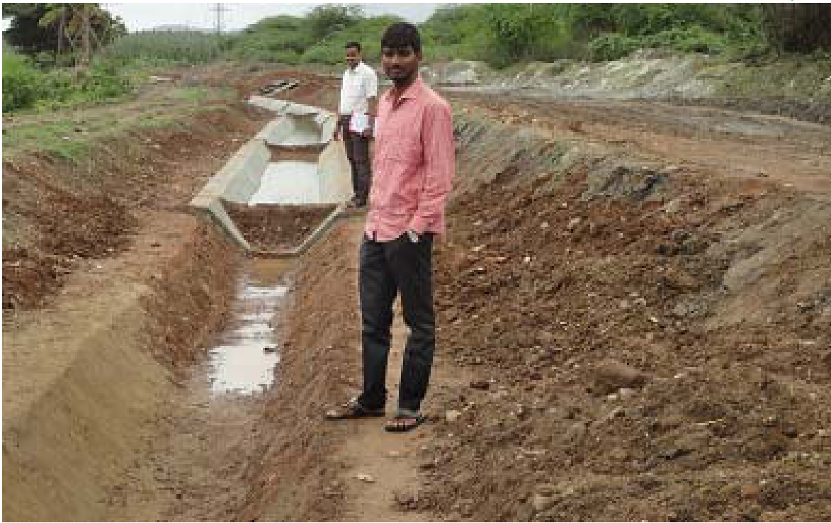
Photo 5: PSC Staff at the construction site to inspect the Silt Disposal Practices of the Contractor – Photograph taken on June 28, 2016
