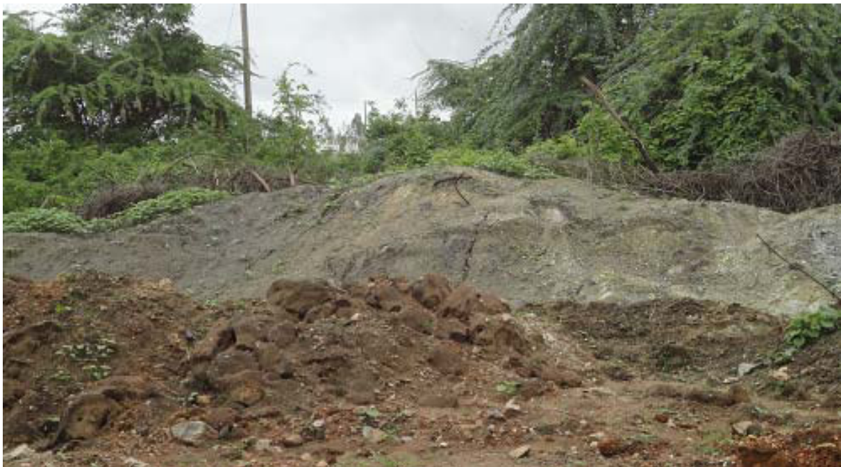
Photo 6: Close-up View of the Disposal of Silt as currently practised by the Contractor – Photograph taken on June 28, 2016
