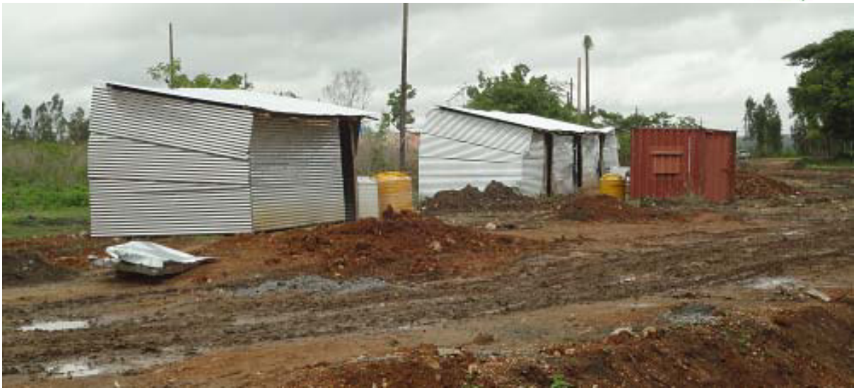
Photo 3: Make-shift Labourer's Quarters provided by the Contractor with Water and Sanitation Facilities
