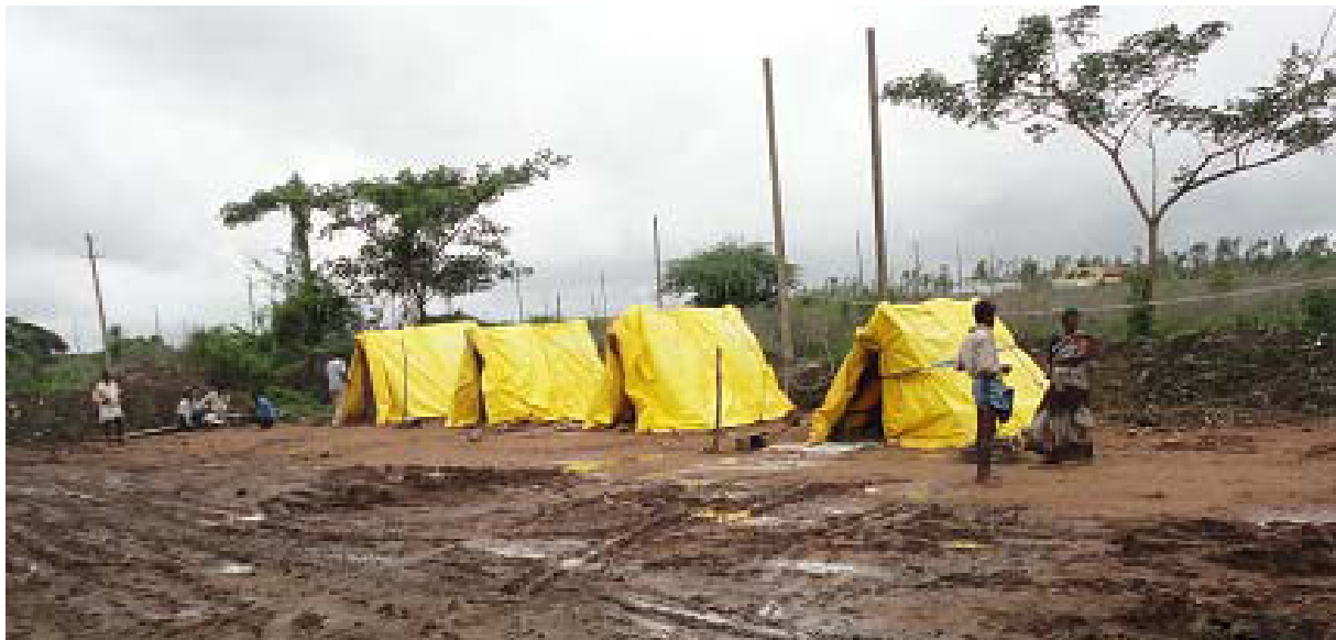
Photo 4: Temporary Shelters provided by the Contractor for labourers to utilise during either a break or temporary halt in construction triggered by natural events – Photographs taken on June 28, 2016
