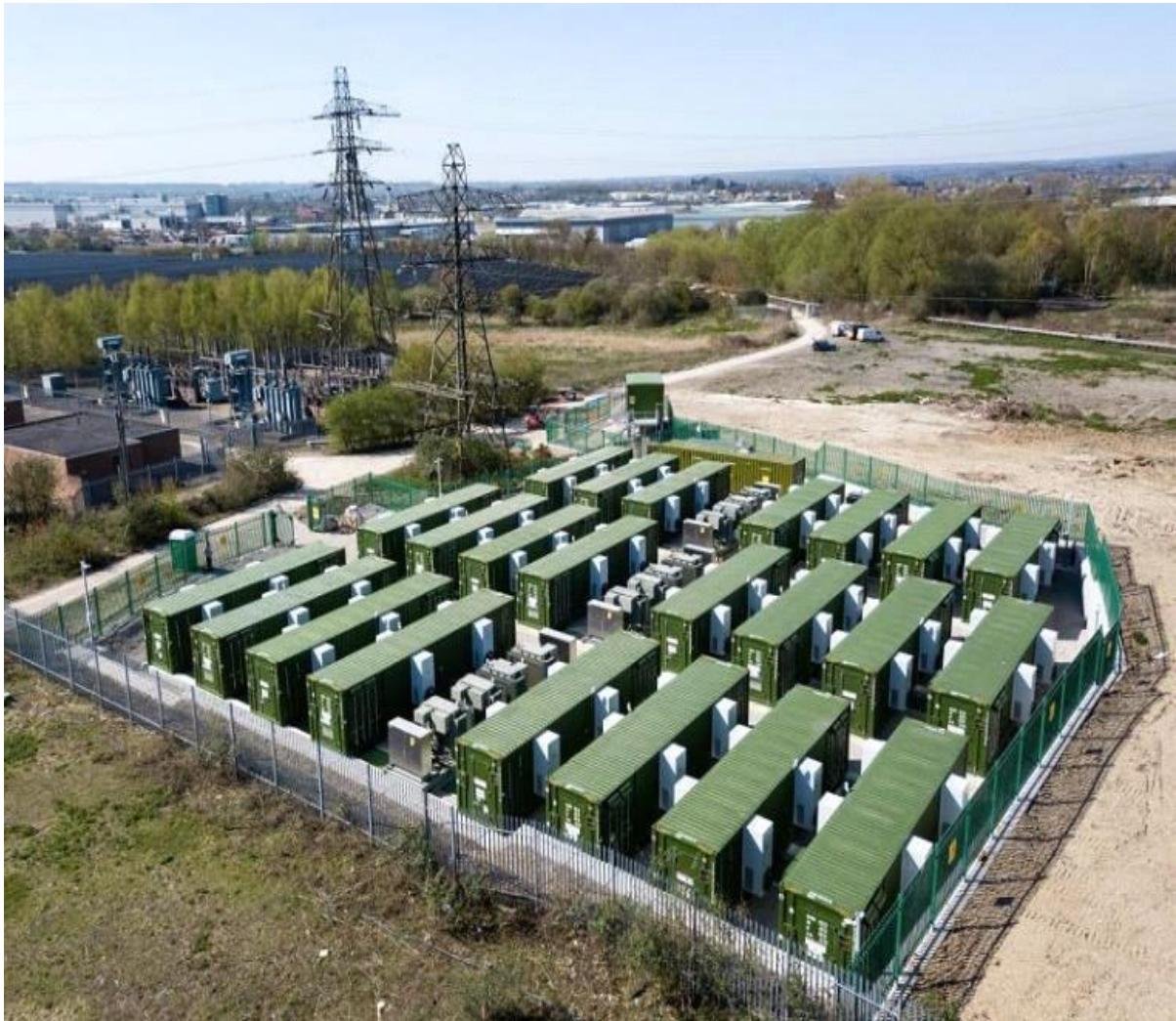
Figure 2-1: Example of a 35 MW BESS unit located at located in Aylesford, UK (Source: Eskom, 2018)
