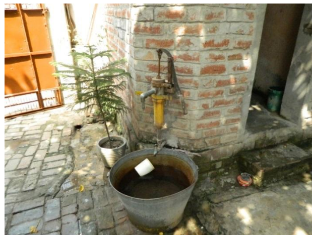
Figure 10.6: Water supply in house in Badial
