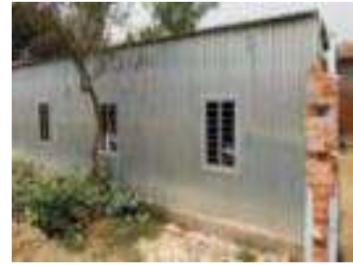
Right picture: A temporary school made of galvanized iron sheets has been constructed, while the concrete school building is not yet finished.
