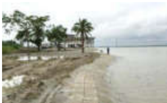
Figure 1-5 Permanent Protection Works
