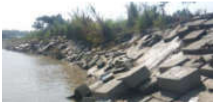
Figure 2-2 Surficial Failure of Riverbank Protection built in 2010
