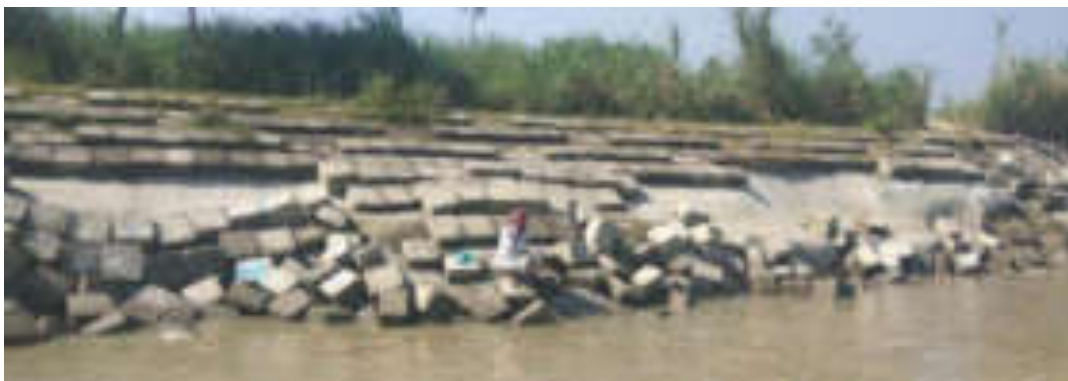
Figure 2-1 Failure of upper slope in Kaijuri
