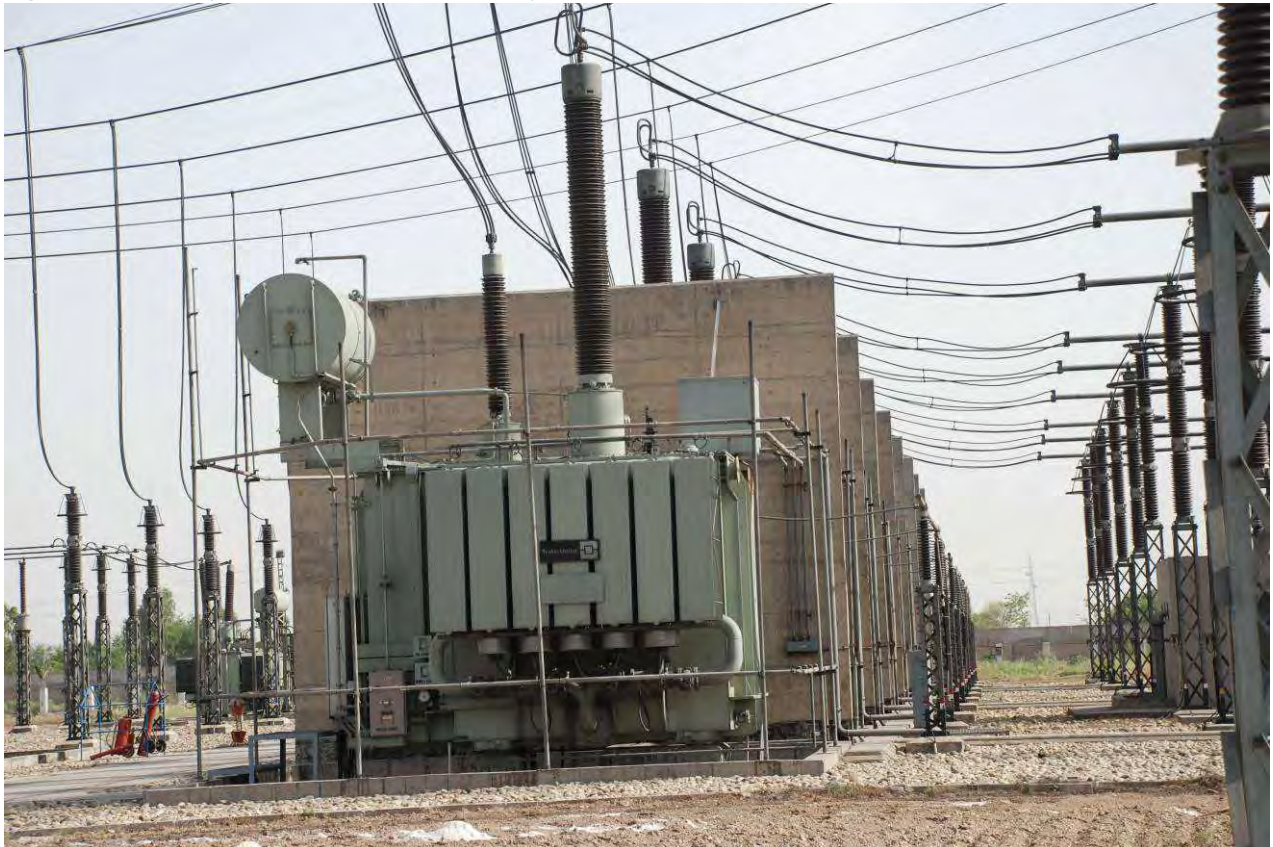
Figure 2.11: Example of Transformer and Switchyard location
