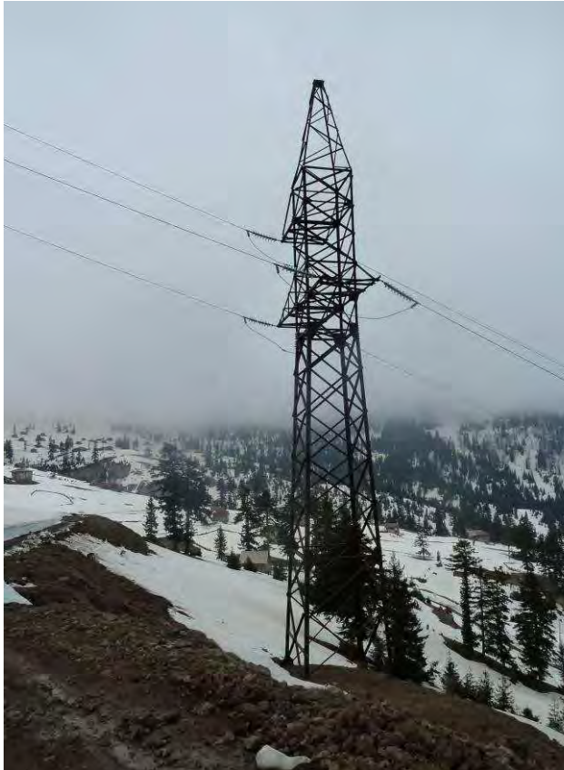
Figure 2.12: Existing 110 kV transmission line
