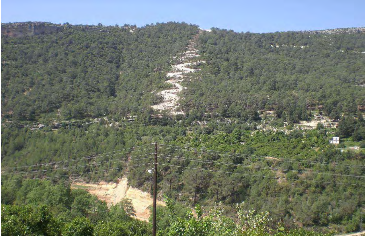
Figure 18.6: Typical view of access road up steep valley side, soon after construction
