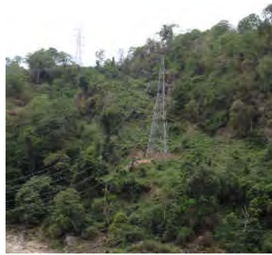
Figure 2-14: Transmission lines at Dagachhu.
