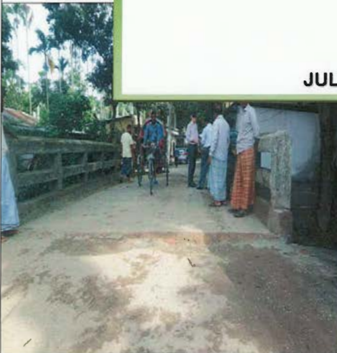
Bhola Pourashava: Damaged Masonry Slab Culvert over Balikandi Khal beside the Town School Field
