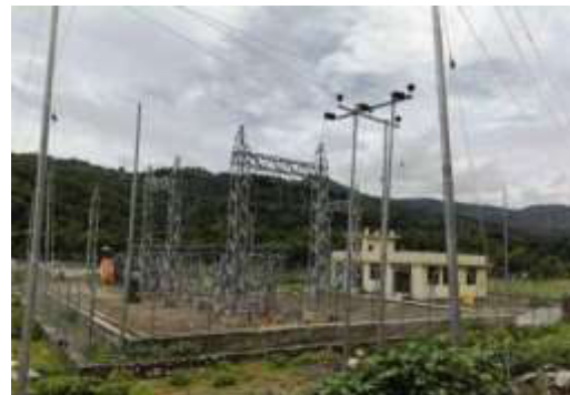
Construction Power sub-station at Damauli
