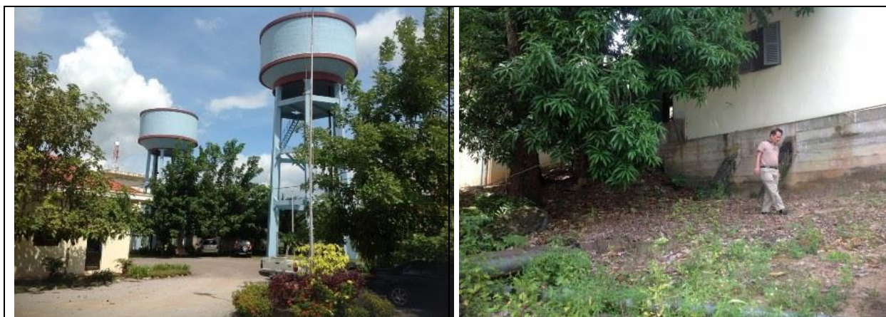
The photo at left shows the two elevated tanks at the entrance of the WTP. The photo at right shows the rear of the intake station at Snom Prampi Village.
