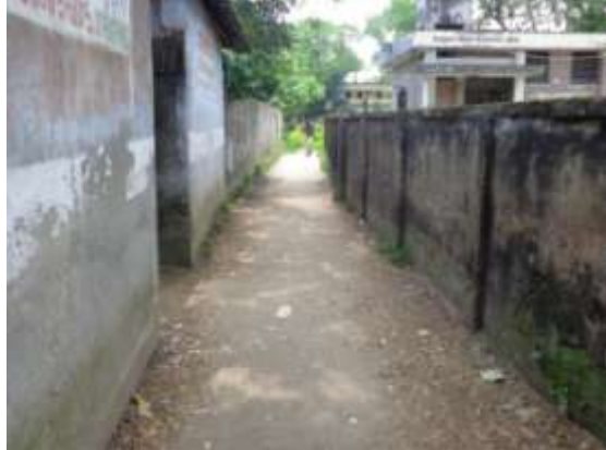
P-12(PDP-38): Construction & widening of road from Govt. Hospital to House Sister of V.P Abdur Rahaman via H/O Ainul Mia by CC. ch. 0.00-330.00m
