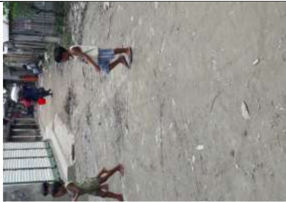
P-14(PDP-91): Construction of road from Volachang New Bazar to Gonnin Para H/O Aziz Mia Via H/O Gafur Mia & Anil Pal road by CC. ch. 0.00-755.00m
