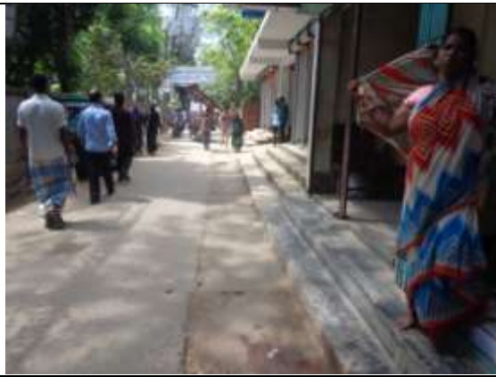
P-09 (PDP-TLCC): Construction of road side RCC drain from Govt. Hospital to the Titas river via S.R Mosque (ch. 0.00-405.00m)
