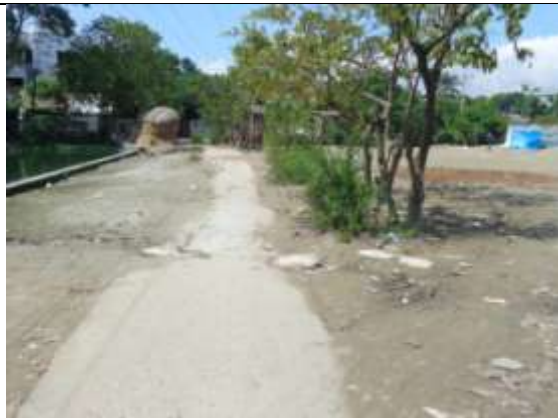
P-19 (PDP-TLCC): Construction of road from Nabinagar Uttarpara Karim shah Mardhasa to Momtola Mosque by CC. ch. 205.00-2130.00m. and Construction of connecting road from Imam Bari to Bhuaiya Kutir Via T&T by CC. ch. 0.00-1060.00m
