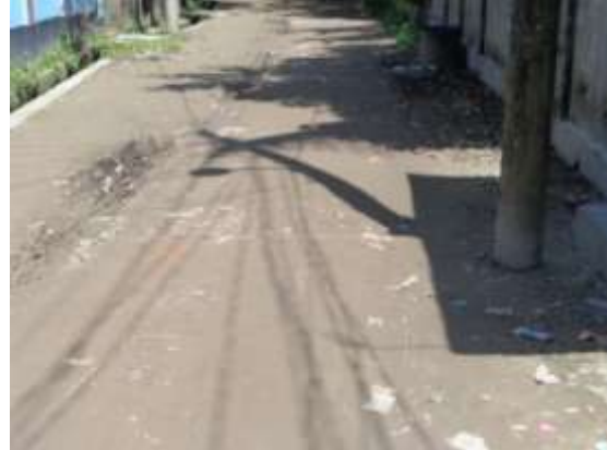
P-13(PDP-22): Construction of road from Nabinagar West para H/O Saidur Commander to Luknath mondir road by CC. ch.0.00-600.00m. Connecting road-1 from H/O Ali Ahamed to H/O Molovi Osman by CC. ch. 00-220.00m. & Connecting road-2 from H/O Manik Bishas to H/O Shek Babi Mosque by CC. ch.0.00-160.00m.
