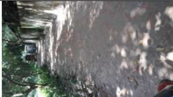
P-16(PDP-71): Construction of road from Narayannpur C&B road to Sha-Shab Bari Mosque by CC. Ch. 0.00-270m and connecting road from Khalek Dr. House to Jahor Mia House via Sha-Shab Bari Mazar road by CC. Ch. 0.00-390.00m
