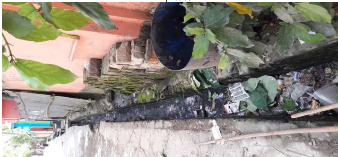
P-21 (PDP-51): Construction of road side RCC drain from Aliabad Tanjab ali market - Aliabad Gopalpur road at the End of Pourashava (ch. 0.00-268.00m).
