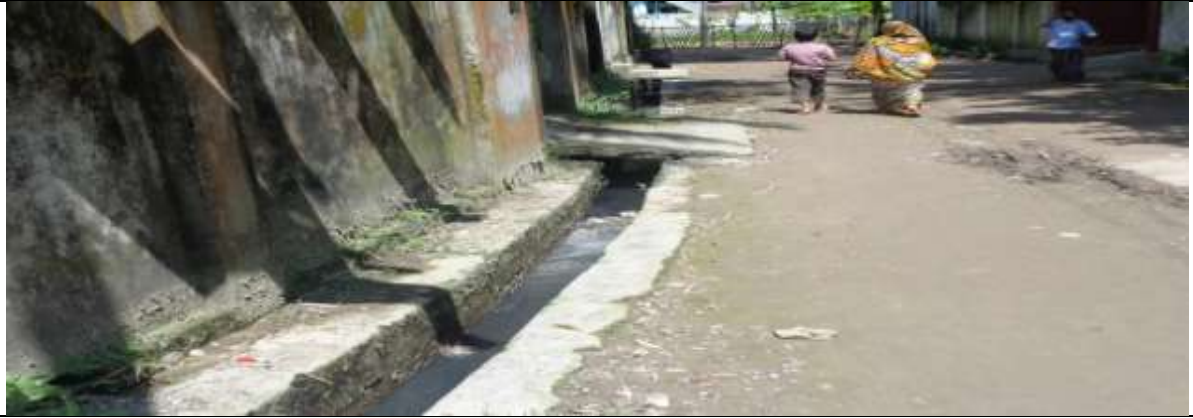
P-18(PDP-22): Construction of road side RCC drain from Nabinagar West para H/O Saidur Commander to Luknath Mondir ch.0.00-530.00m and Connecting drain-1 from H/O Ali Ahamed to H/O Molovi Osman. ch. 00-220.00m. & Connecting drain-2 from H/O Manik Bishas to H/O Shek Babi Mosque. ch.0.00-160.00m.
