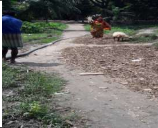
P-07(PDP-TLCC): Construction of road from Dolabari C & B Road to Nabipur Govt.Primary school Via East side of Kali Mondir by CC. ch. 0.00-412.00m.
