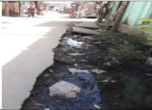
P-10(PDP-TLCC): Construction of New RCC drain Majikar Nupur Cinema Hall to Titas river via H/O Moti Mia and CNG stand. (ch. 0.00-470.00m).
