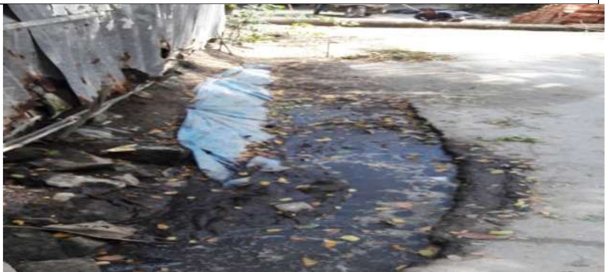
P-11 (PDP-TLCC): Construction of road side RCC drain from C & B road to Sattar Mia house mosque via Lil Mia Bapari (ch. 0.00-520.00m).
