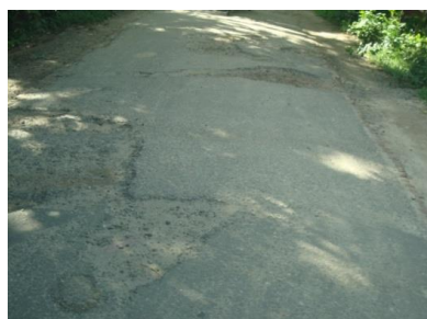
Narrow PS road with a bad worn-out surface, displaying a lack of routine maintenance
