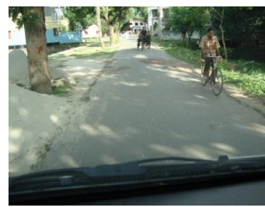
Another PS road, showing a surface damage ahead, which is another example of maintenance shortfall
