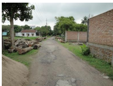
A PS-road with very badly damaged surface and displaying poor maintenance
