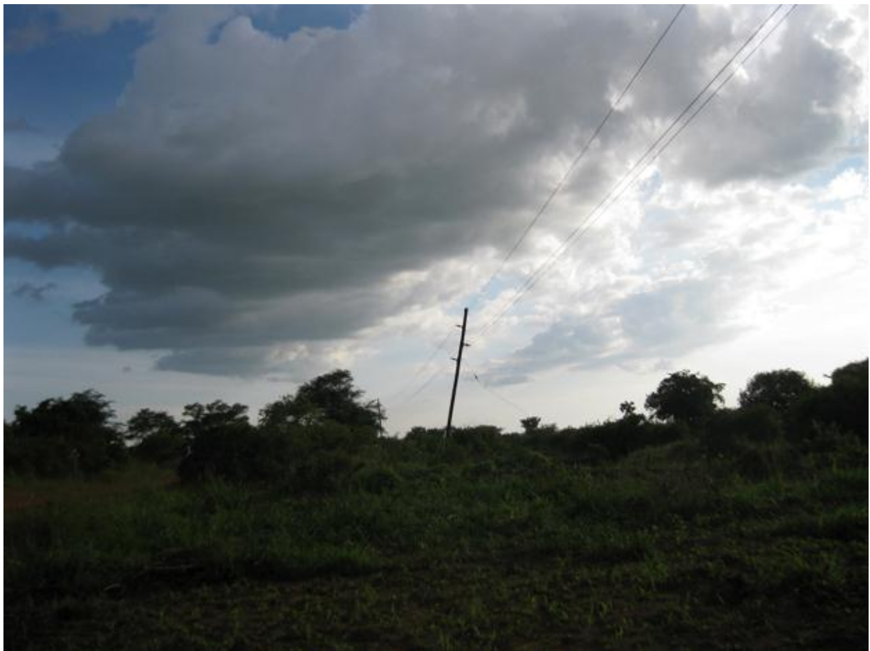
Plate 6.1: Sagging electric pole
