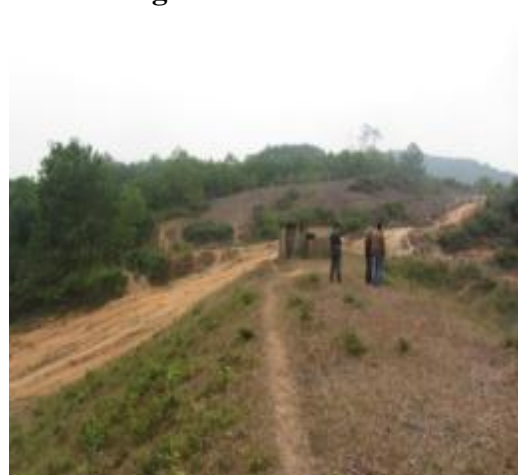
Figure 2-5: Left shoulder is eroded
