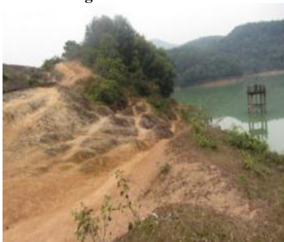
Figure 2-4: Left shoulder is eroded by rain
