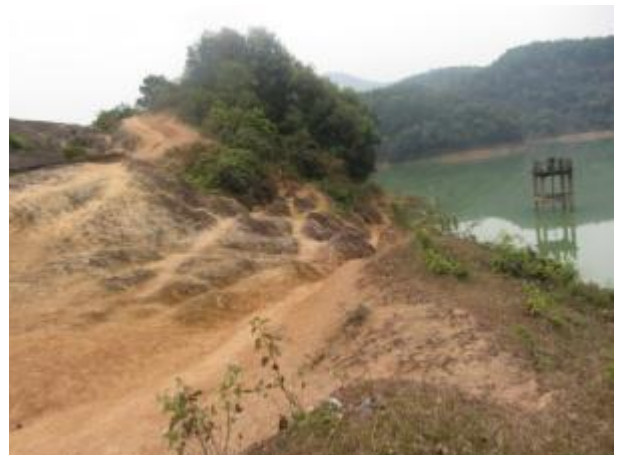
Image 4: Eroded left shoulder of the dam caused by rain
