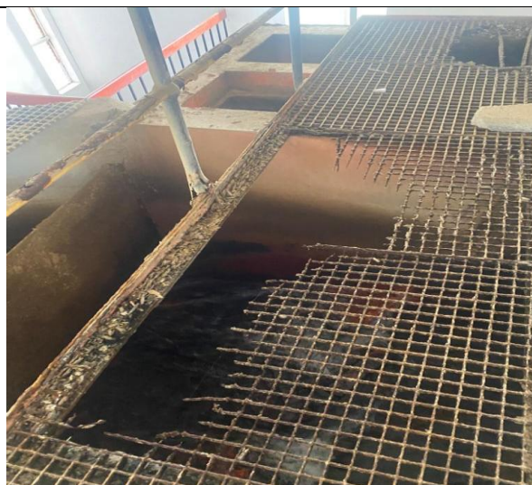
Intake point needs refurbishment
