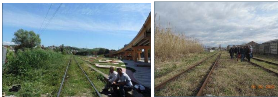
Figure 2-27_Neglected drainage channel partly filled with sediments and covered of vegetation ( pragmites australis ). Left: km 5+180 (Plepa); Right: Shkozet station
