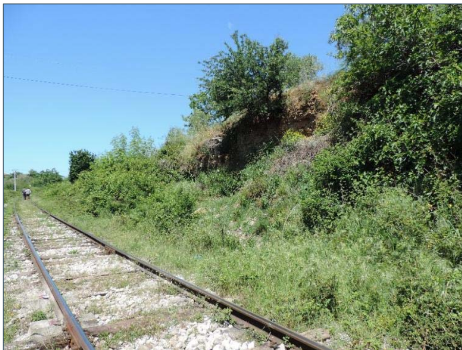
Figure 2-28_Drainage channel filled with sediments because of the lack of maintenance and retaining walls (Gose Vogel Village area)
