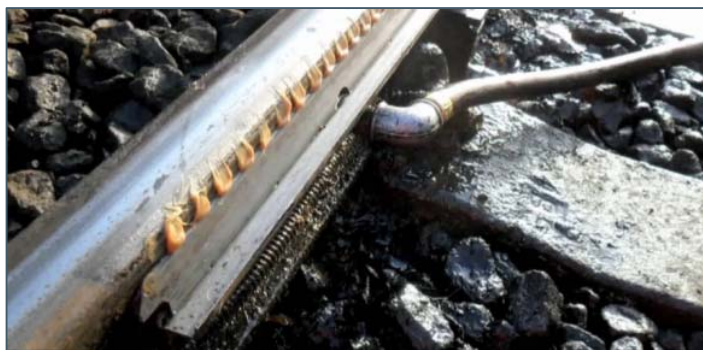
Figure 6-4_Track-side lubrication system
