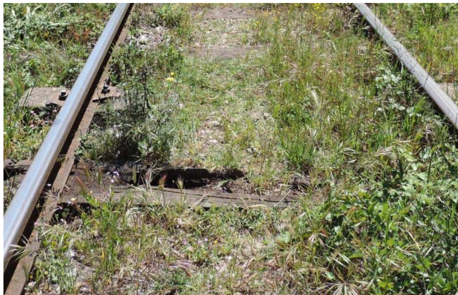
Figure 2-9_Damaged timber sleeper at the northern entrance of Rogozhine tunnel
