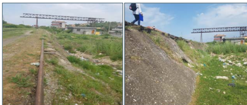
Figure 2-22_Sliding of retaining wall - Kavaje
