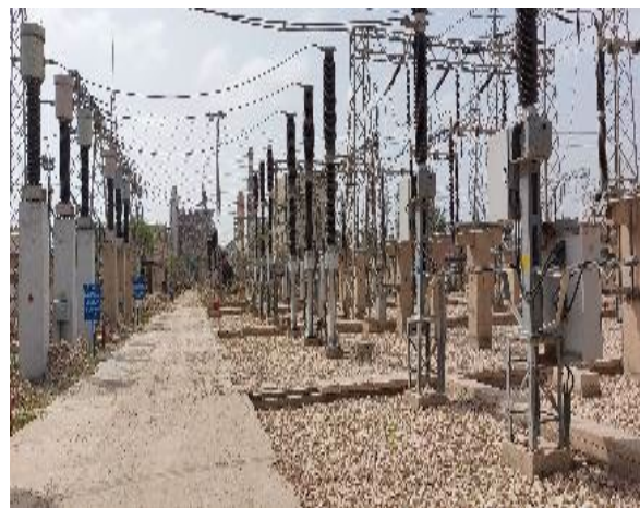
220 kV Switchyard at the GS
