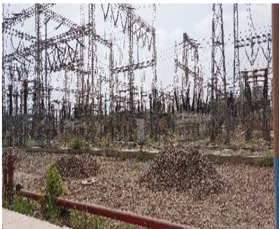
220 kV Switchyard at the GS
