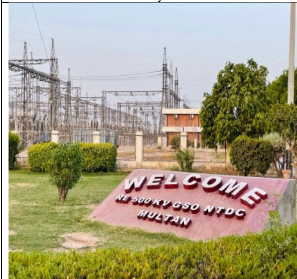
View of Switchyard area
