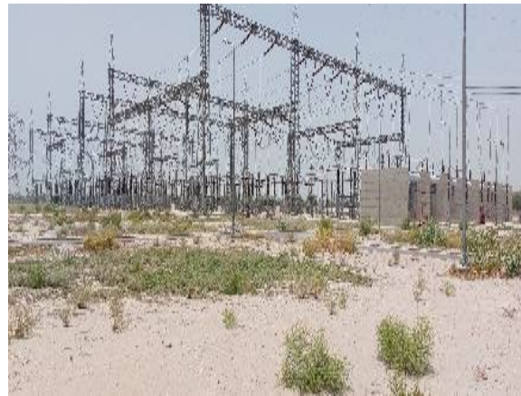
View of Switchyard with Transformer Bay
