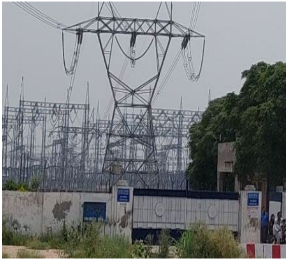
Entrance to Sheikhpura GS
