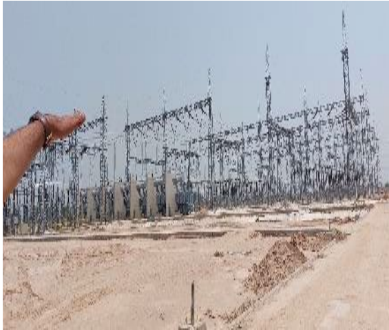
View of Transformer Bay and Switchyard
