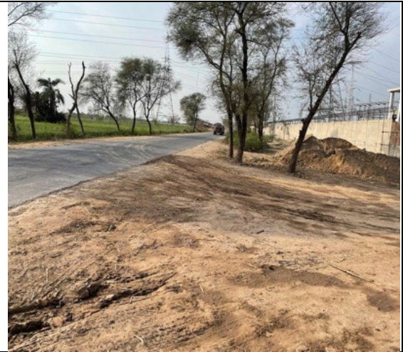
Another view of front site towards Painsra – Bhawana Road of 500 kV, 220kV & 132kV Grid Station (Faisalabad West)
