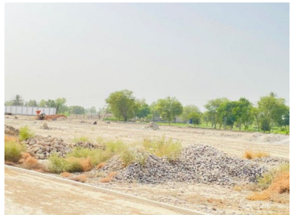
Boundary wall is under construction and agricultural area is visible in the surrounding
