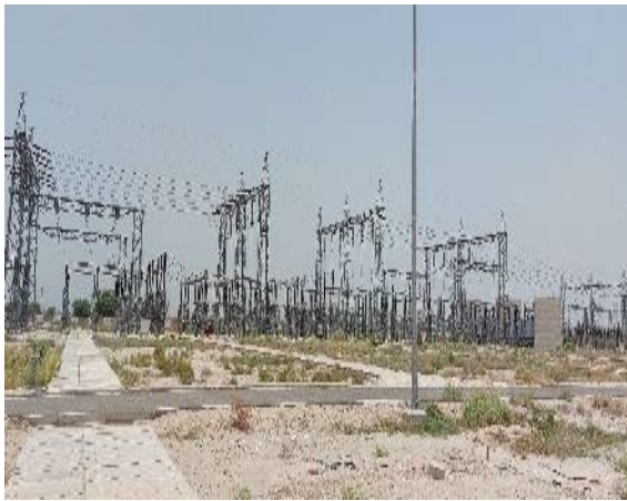
View of Switchyard
