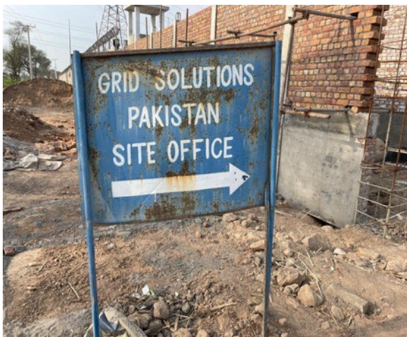
Signboard displaying in the front of 500 kV, 220kV & 132kV Grid Station (Faisalabad West)
