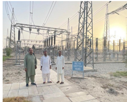
View of 132 kV switchyard at G/S
