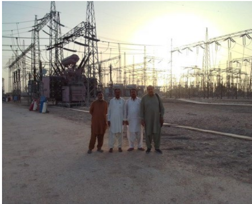
View of switchyard at the G/S & Scope of work
