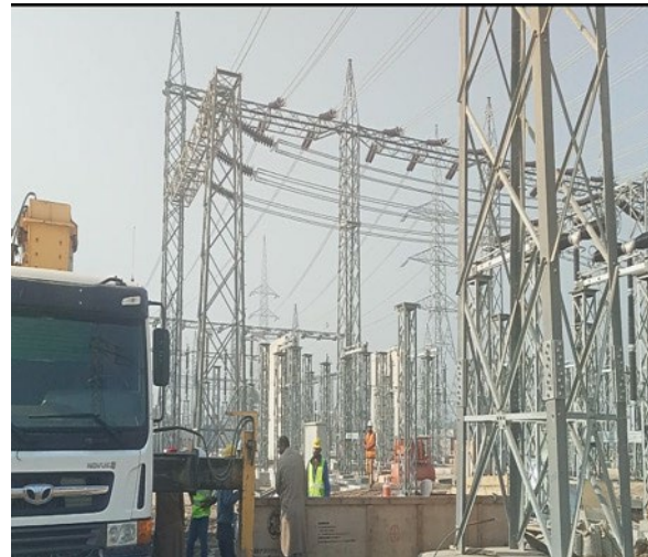
View of the ongoing construction work in the 500 kV, 220kV & 132kV Grid Station (Faisalabad West)
