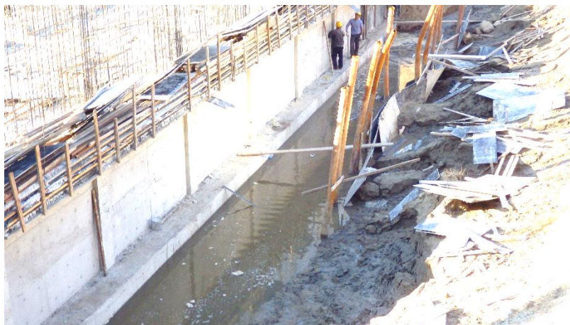
Figure 67 Working in damp condition around a pumping station
