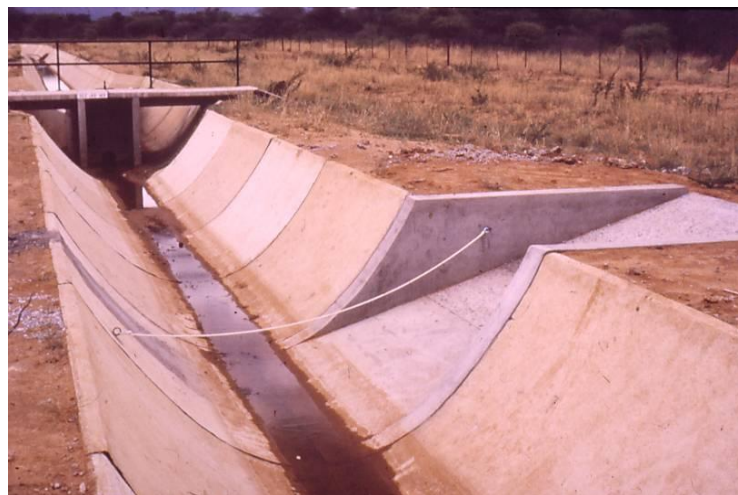
Figure 76 Inefficient escape structure
