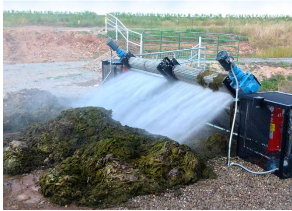
Figure 88 Small scale automatic debris removal screens
