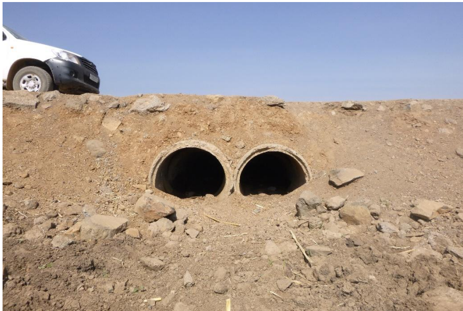
Figure 83 Inadequate culverts in an earth dike across a seasonal river
