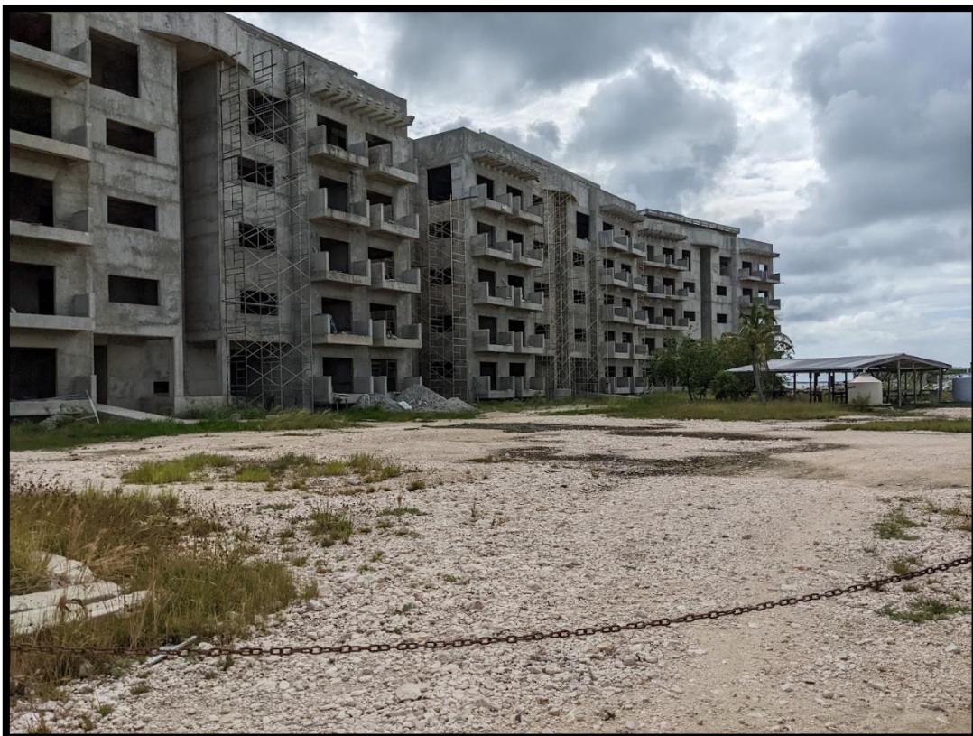
Figure 21 - Final point of south main. Residential complex under construction (Photo: PlanEHS, Nov. 2022)
