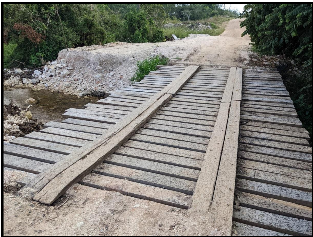
Figure 29 - Drainage canal crossing in easternmost proposed main in Harmonyville (Photo: PlanEHS, Nov. 2022)
