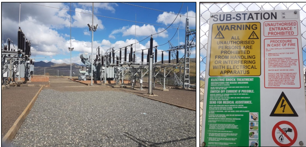
Figure 4.40 Typical Substation (Ha Lejone)
