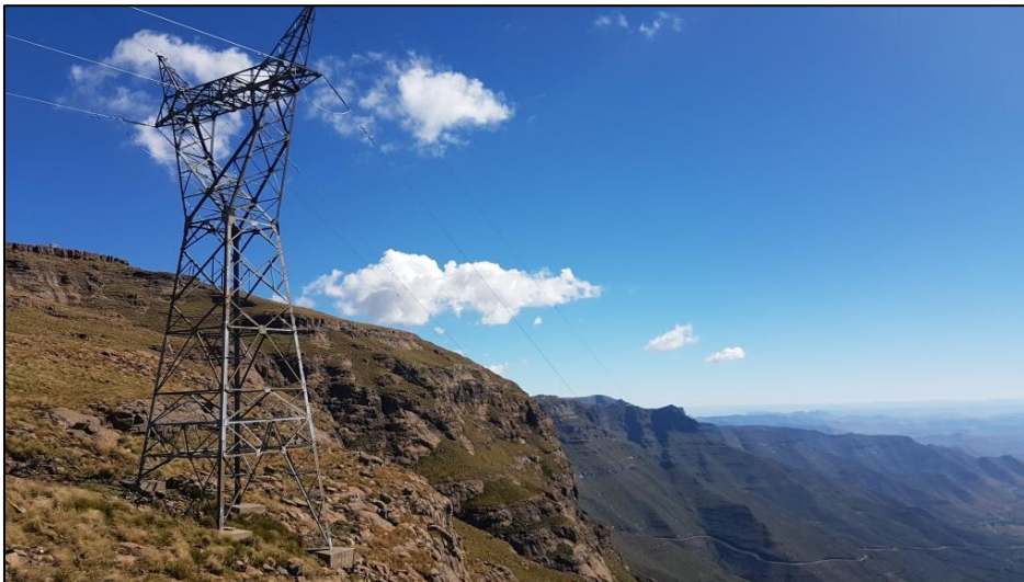
Figure 4.35 Eskom Type 247 Pylon (132kV) at Bend Point (Deviation Pylon)
