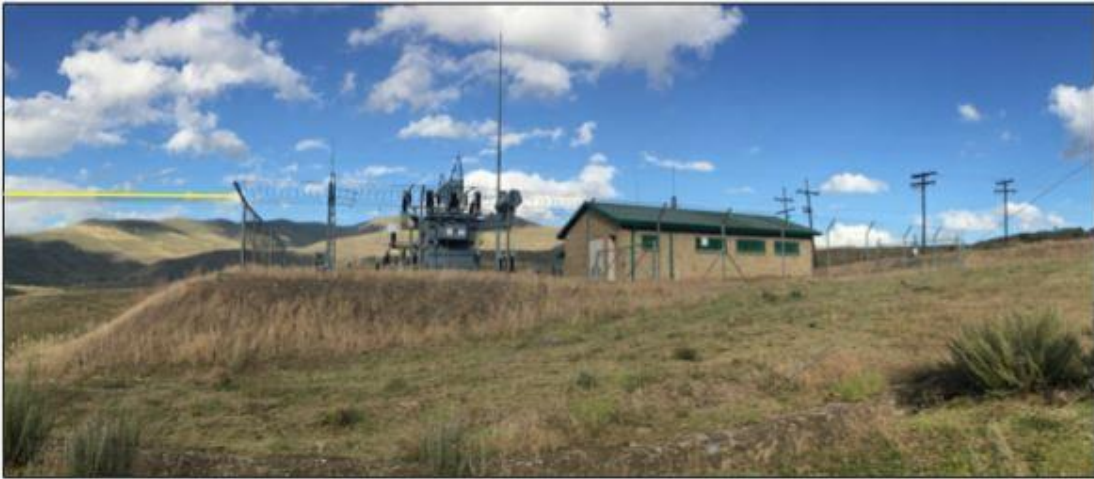
Photo Point 1: View of the Matsoku Intake substation. This will be expanded towards the left of the picture to accommodate the increased capacity requirement and additional powerlines.
