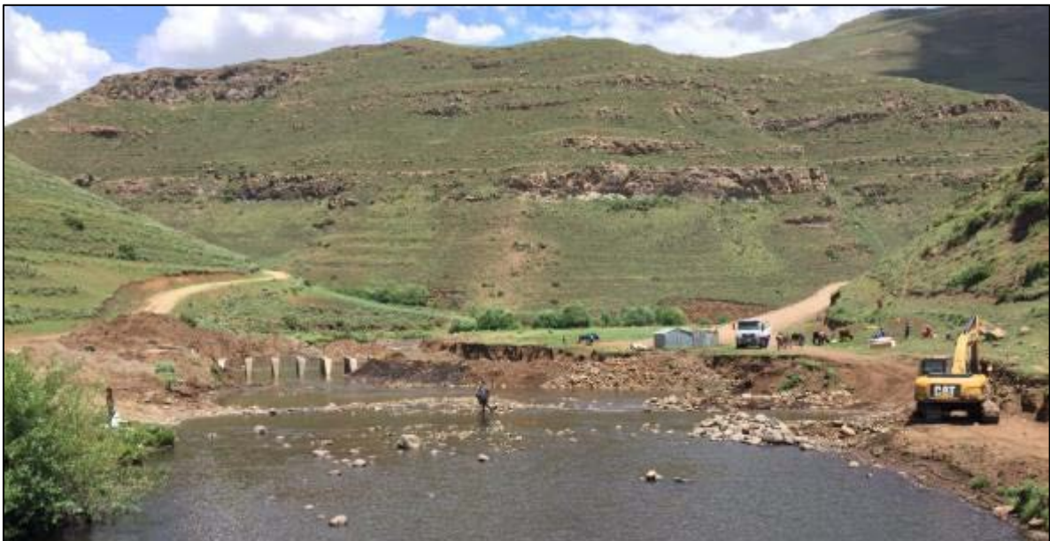
Figure 12.14 Construction Underway on a Bridge on the Matsoku River, Showing River Bank Disturbance
