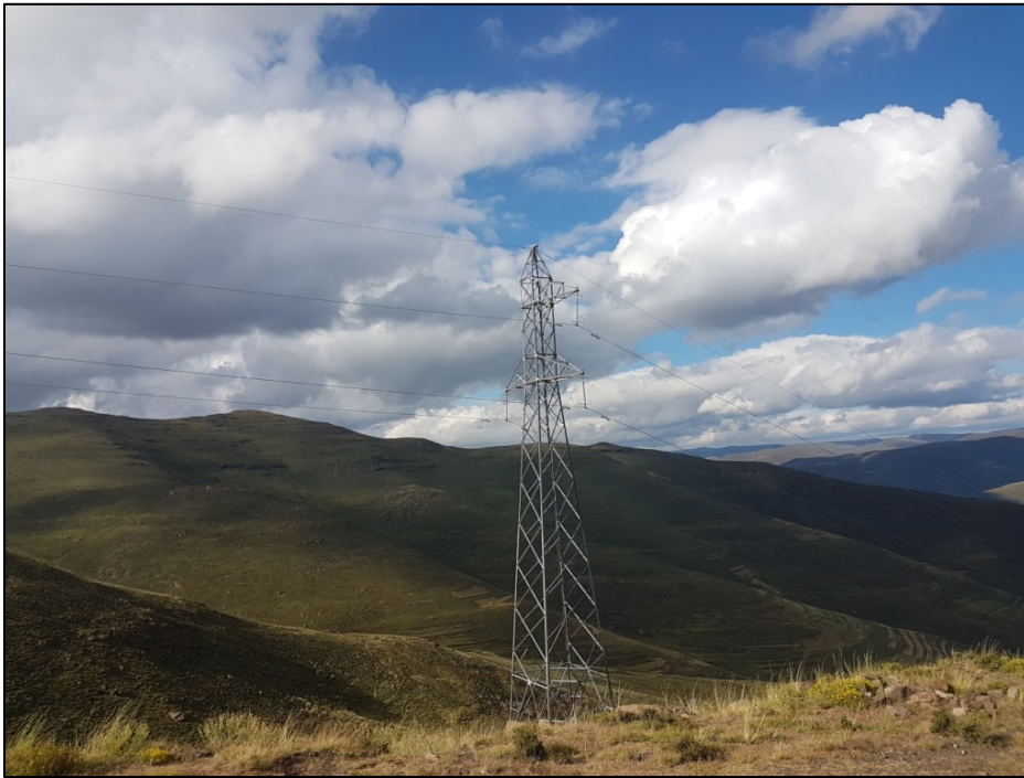
Figure 4.34 Eskom Type 247 Intermediate Pylon (132kV)
