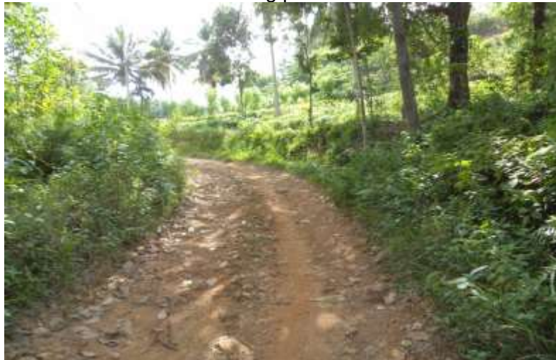
Plate 2: Poor gravel road Section through 0+200 - 0+700km
