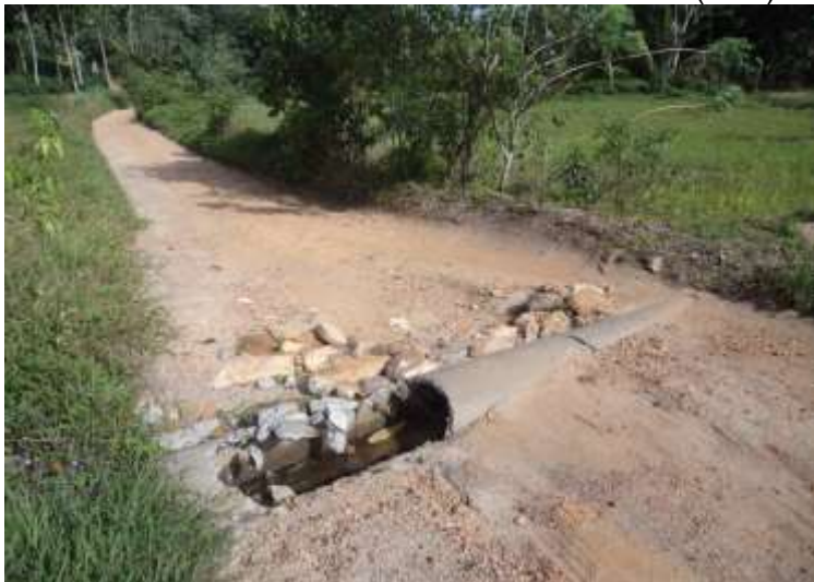
Plate 8 : Poor cross drainage structures - 3+400 - 3+500km
