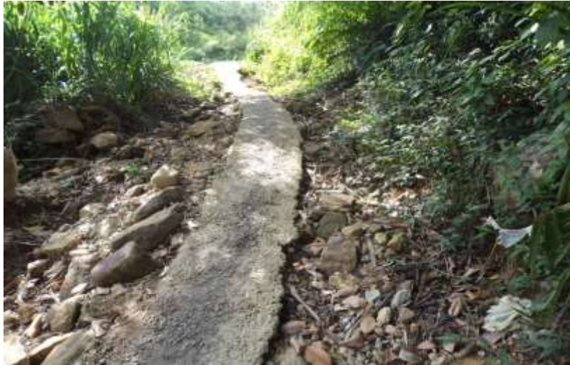
Plate 4: Road at 2+800 - a dilapidated section
