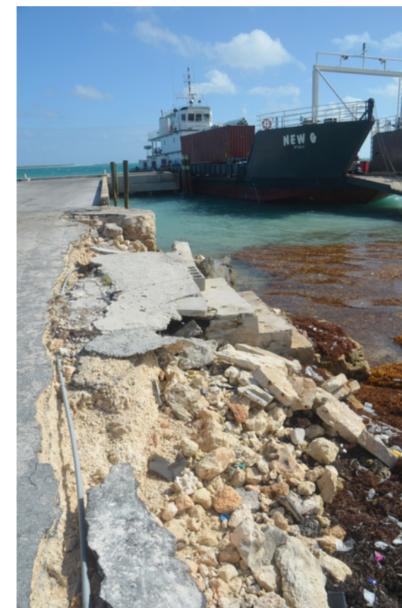
Photo 2- Damage to a dock on Long Island
