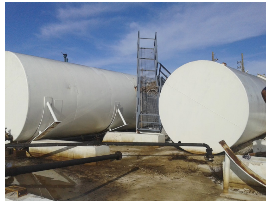
Photo 3- Damage to fuel tanks
