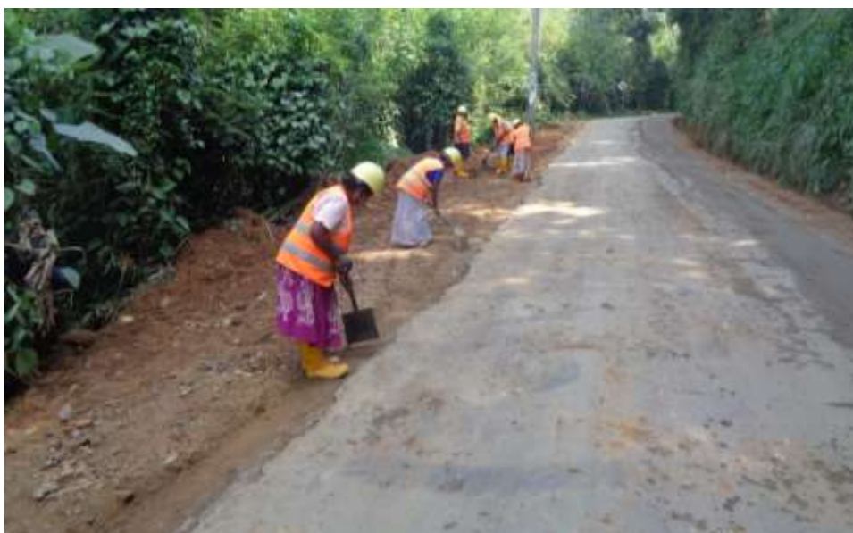
Figure 6.6 Female workers involved in road construction work at Athiliwewa Junction to D.S. Gama Road (MO6 package)
