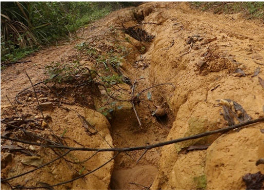
Road erosion on a slope section
