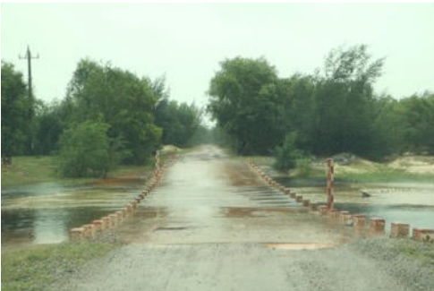
Flooded spillway at Km7+784 - Section 1
