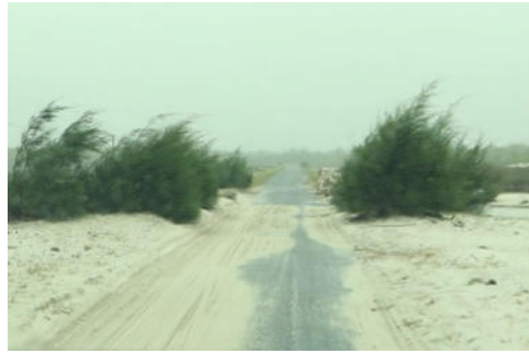
Sand covered the road in Section 3
