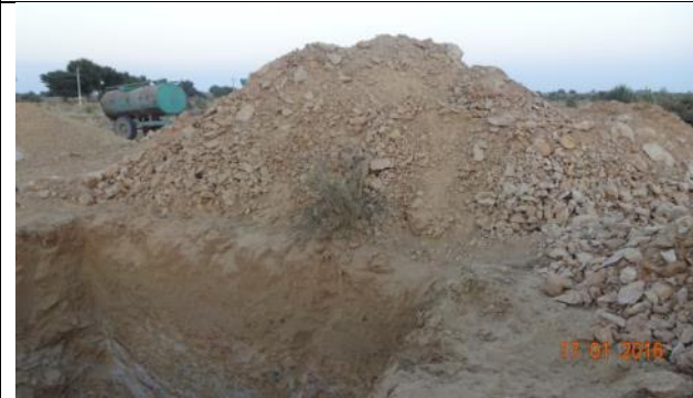
1.10 Stacked topsoil besides a tower foundation pit very near to the edge.
