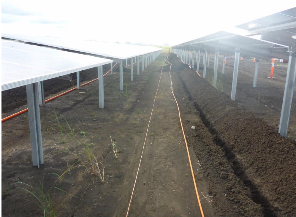
▲ Photo 9 – Installation of solar PV arrays and electrical conduits at Henderson – Fighter 1 solar PV site (2015).
