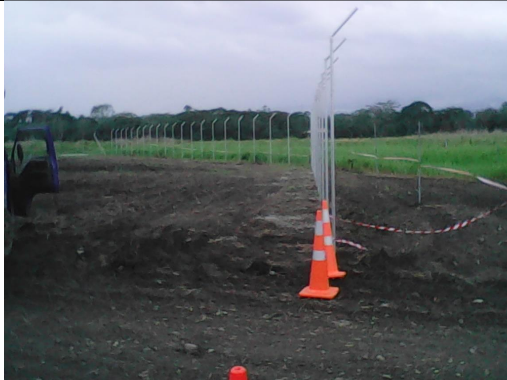
▲ Photo 8 – Installation of chain link security fencing around the perimeter of the Henderson – Fighter 1 solar PV property (2015).
