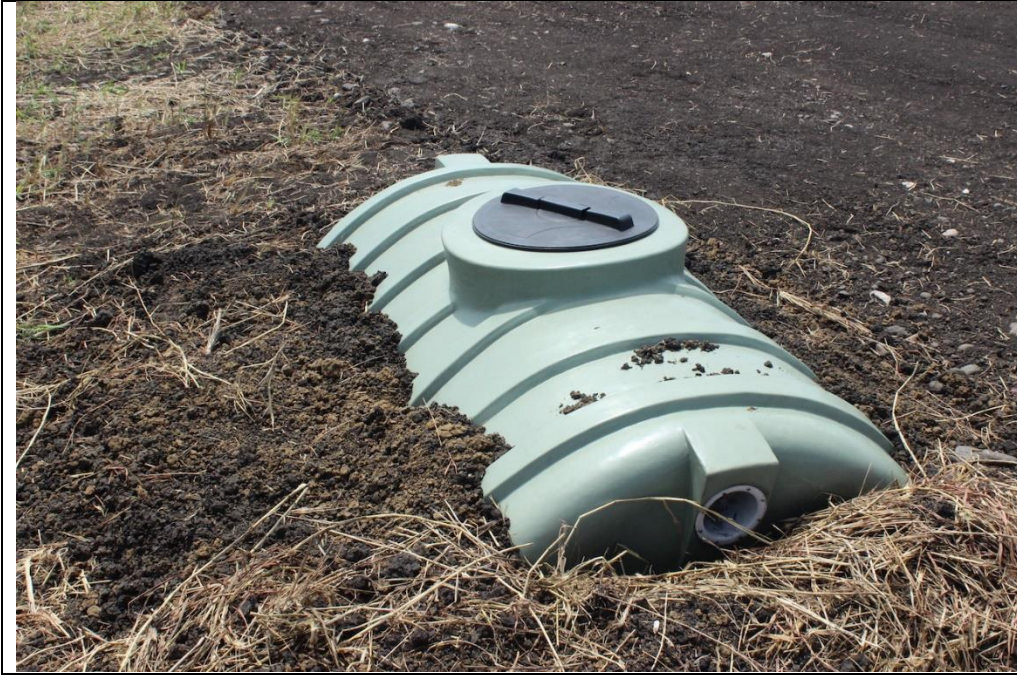
▲ Photo 7 – Installation of septic tank for treating sewage wastes generated from construction and operating staff (2015).
