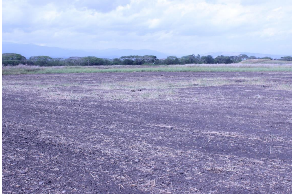
▲ Photo 4 – Pre-construction site clearing and grading in preparation for installation of solar PV arrays and ancillary equipment (2015).
