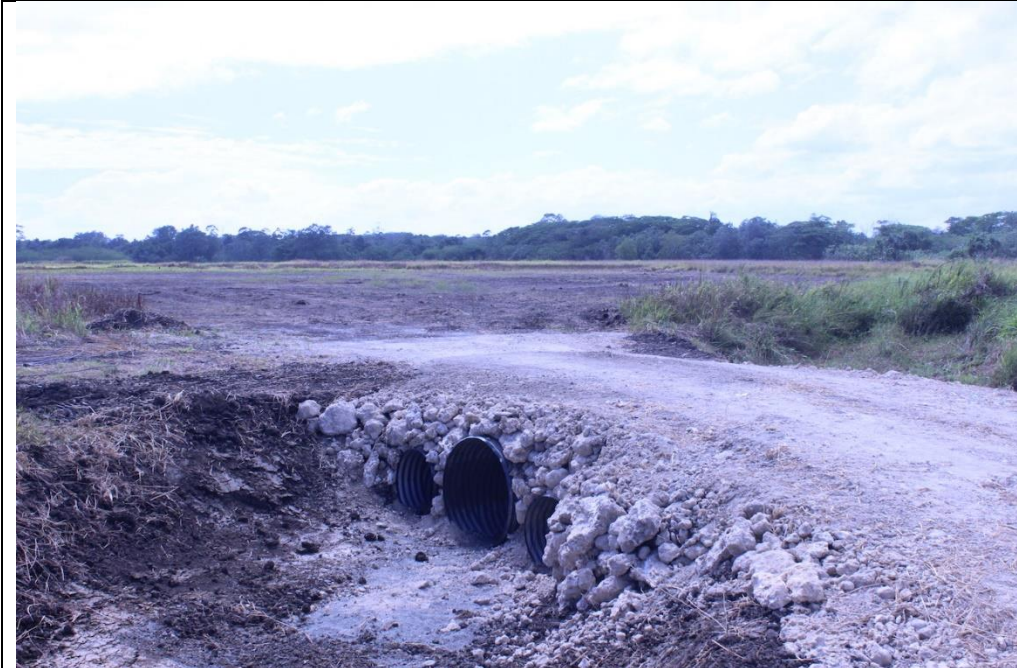
▲ Photo 6 – Culverts installed under access road at entrance to Henderson – Fighter 1 solar PV site on Southwest end of the property (2015).
