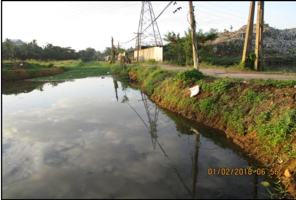
Existing View of the Upstream of the Pipe Culvert Across the Main canal (Opening is not adequate) - Minimum requirement is 30 m span bridge
