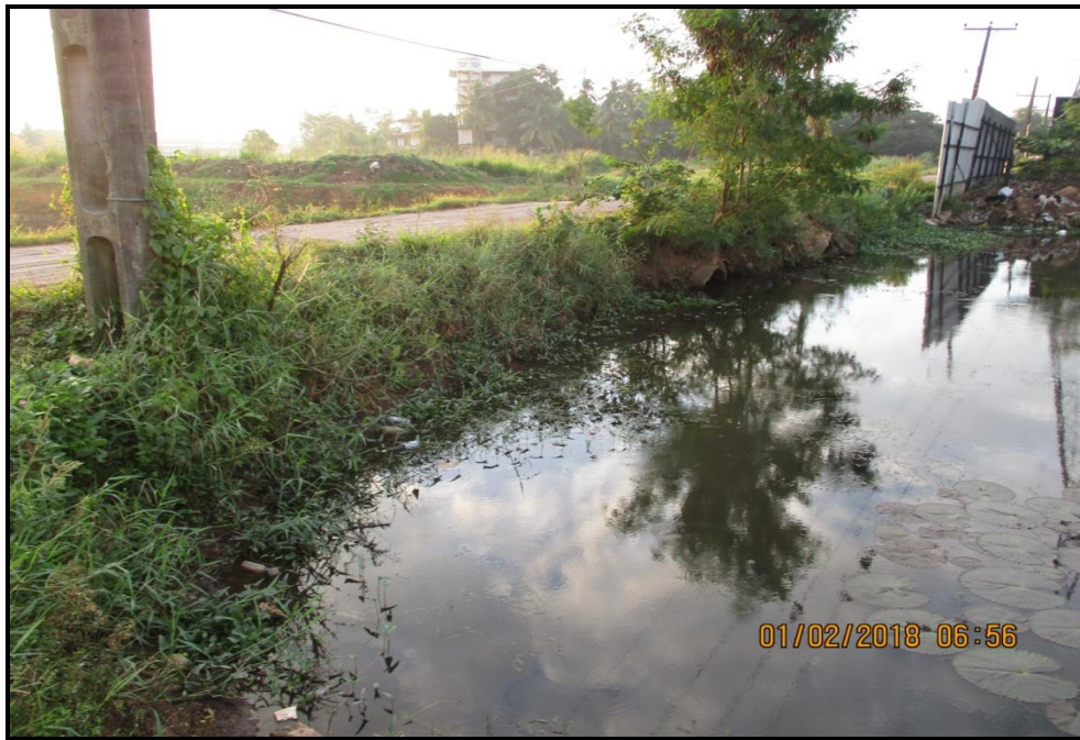
Existing View of the Downstream of the Pipe Culvert Across the Main canal (Opening is not adequate) - 30 m span bridge
