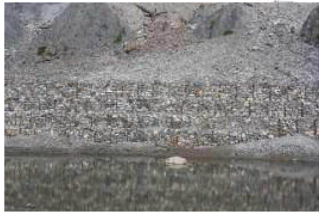
Fig. 1.11 Boundary area erosion (Source: HCP site photos)
