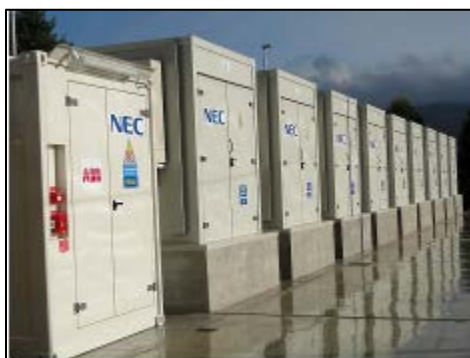
Figure 12: Example of 2 MW lithium ion battery system.
