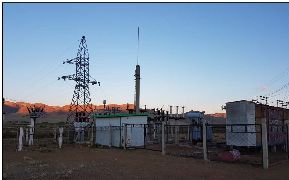
Figure 15: Aldarkhaan 35/10 kV substation.
