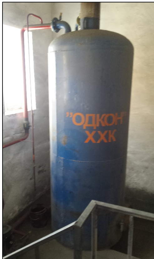
Figure 30: Khovd Kindergarten Boiler.
