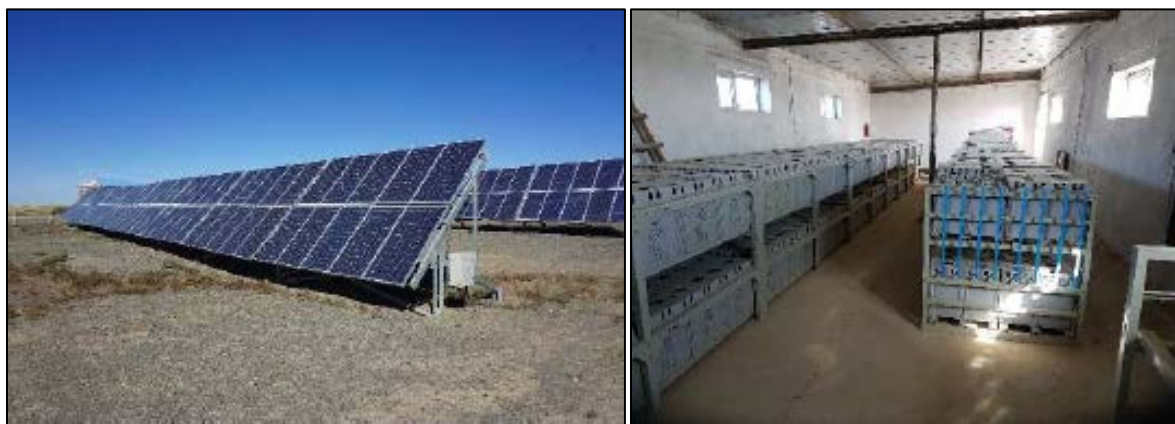
Figure 22: Altai Soum existing 200 kW PV farm.
