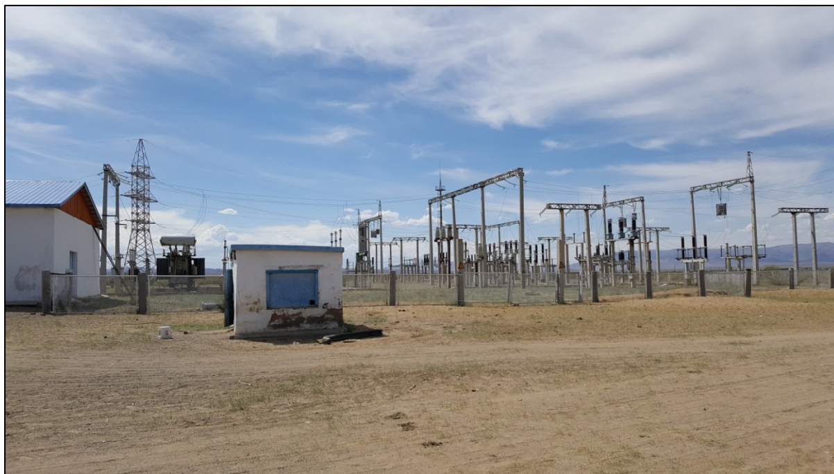
Figure 6: Umnugovi 110/35/10 kV substation.
