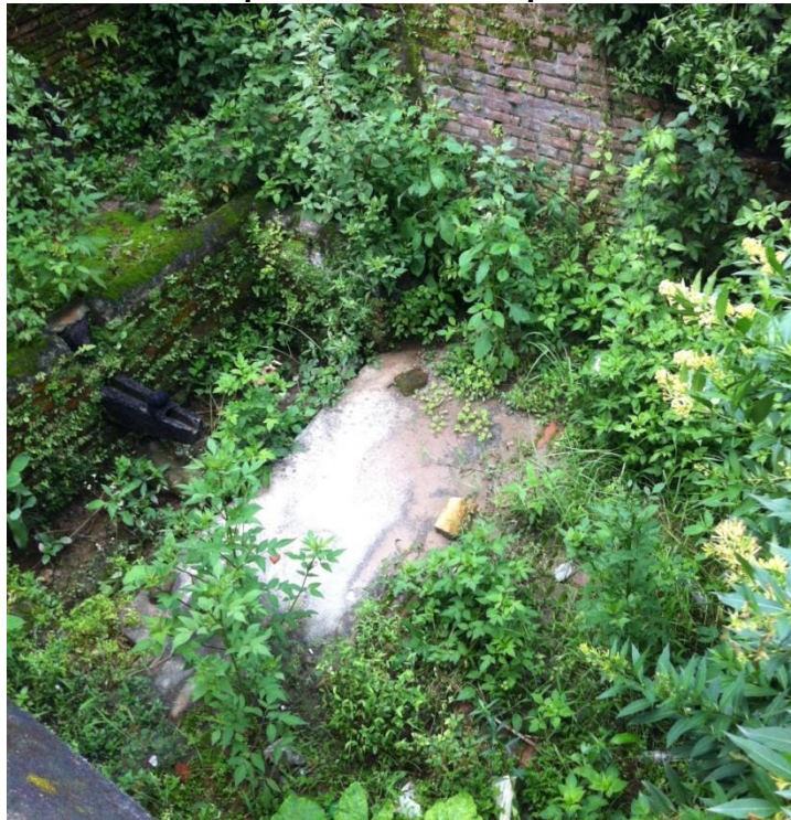
Photo 4: Non Operational Water Spout at Lainchaur
