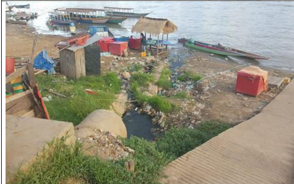
Figure 25b: Nakasang grey water drainage discharge into the Mekong to be extended
