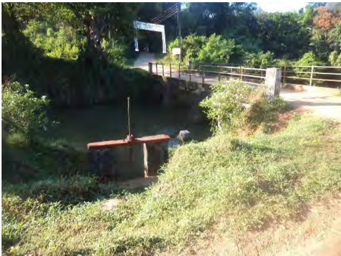
Overlooking the bridge and intake of turnout which are to be rehabilitated
