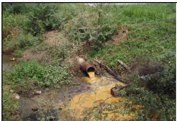
OUTLET OF THE INDUSTRIAL WW PIPE (10") FLOWING SOUTH TO MCDC POND SYSTEM. BOD TESTED WAS >6,700 MG/L
