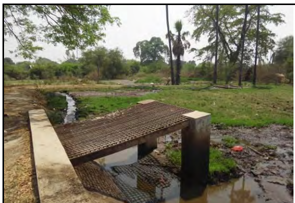
DISCHARGE FACILITY FOR TRUCKS AT THE OXYDATION POND
