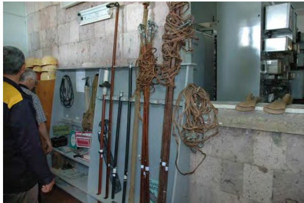
Photo 4-9: Basic safety equipment as helmets, gloves, tools for working under high voltage and signs at the substations
