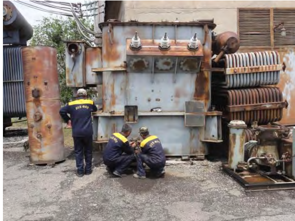
Photo 9-1: Discarded equipment is used for storage of old and/or spare oil. This old equipment is often leaking.
