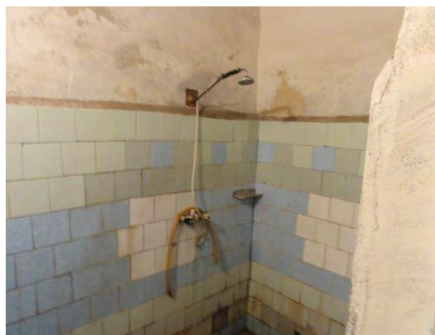
Photo 4-12: If washing facilities exist, they are badly maintained
