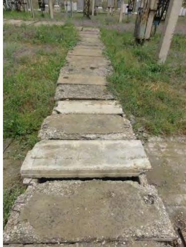
Photo 4-1: Cable ducts used as pathways are often broken and show holes
