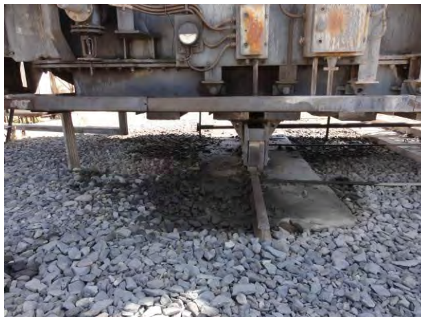
Photo 4-16: Leaking oil pollutes the gravel below an autotransformer
