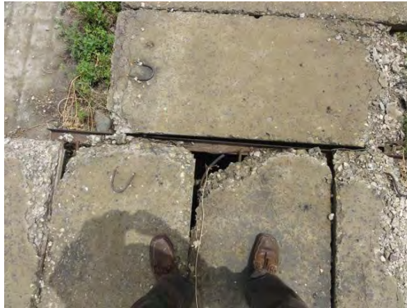
Photo 4-2: Cable ducts used as pathways are often broken and show holes
