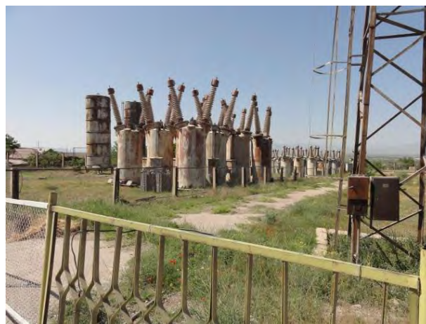
Photo 4-13: Old circuit breakers stored at substation site sometimes since decades
