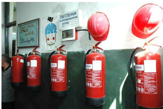
Photo 4-7: Sufficient well maintained powder based fire extinguisher were available inside the control buildings of all substations
