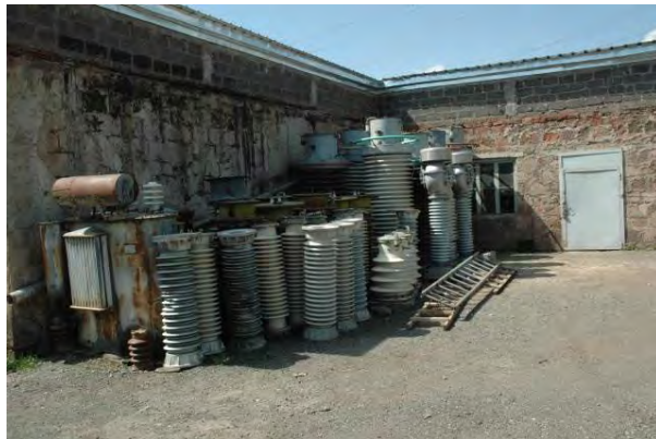
Photo 4-15: Ceramic waste stored at a substation site
