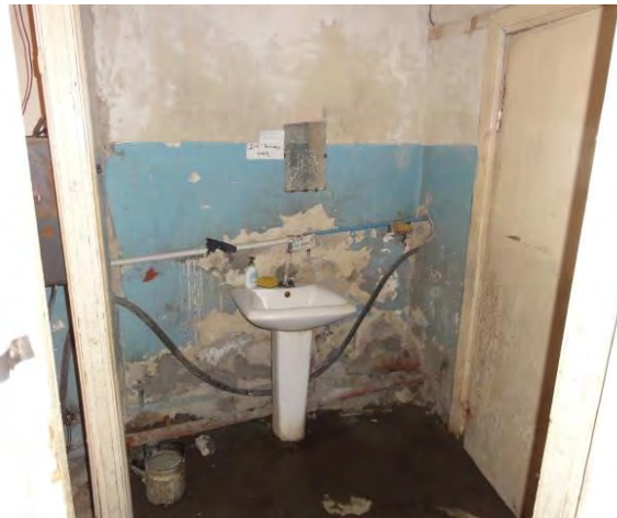
Photo 4-11: If washing facilities exist, they are badly maintained
