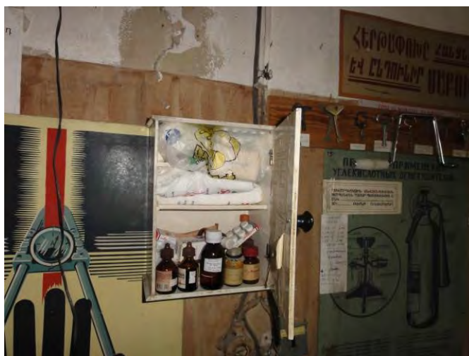
Photo 4-5: First aid kits as available at substation sites are partly maintained very poorly
