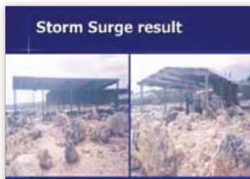
Photo12: Strong storm surge damaging Nafanua Harbour, MoW, 2003.
