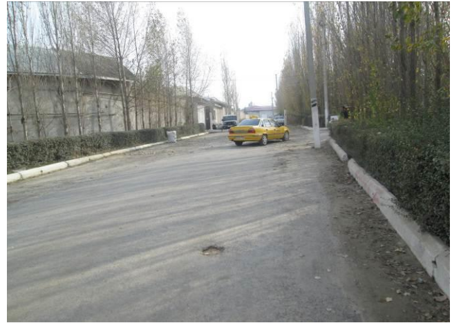
Pic.4. Near the Hospital-1. Sewerage pipes will be laid under this road.
