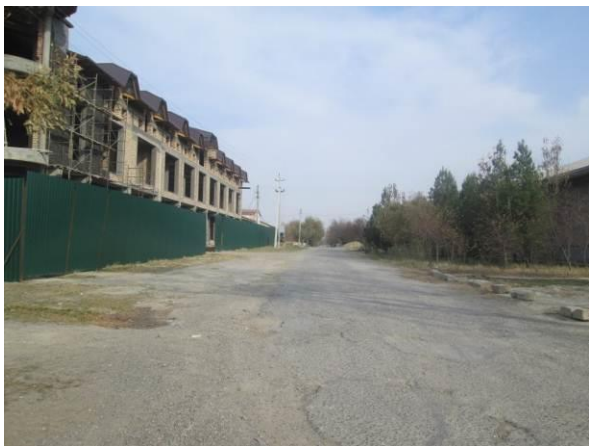
Pic. 7. Street-7 where sewerage pipes will be laid in the middle of the street.
