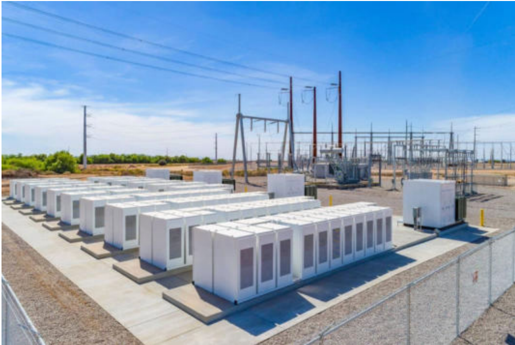
Example completed BESS facility
