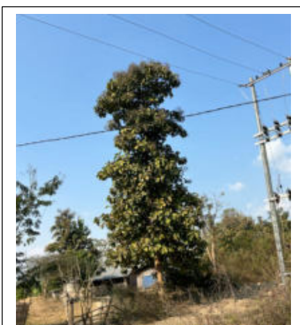
Figure 65: Distribution line in SPP
