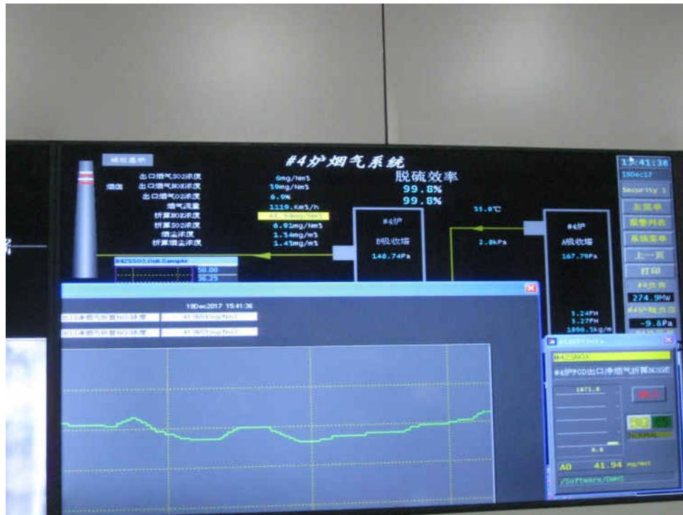
Figure 20: Zhangqiu TPP monitoring system showing real-time CEMS data
