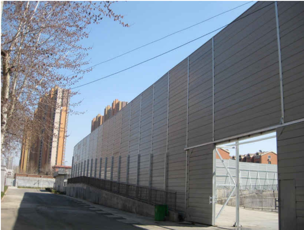
Figure 8: Dongxin TPP noise barrier
