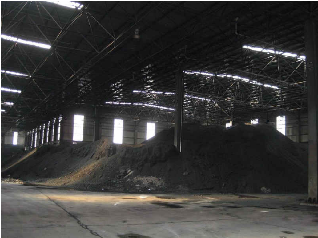
Figure 6: Coal storage room, Dongxin TPP
