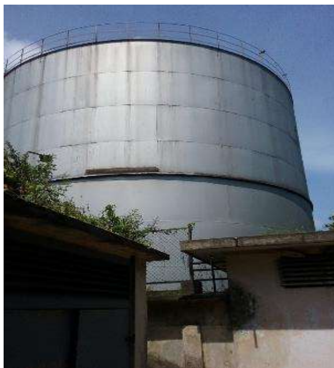
Photograph No. 04 – Oil Tanks Ch- 1+784
