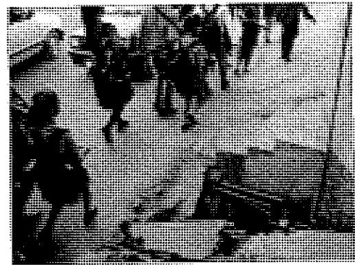
2. Side steps intrude into the public right of way and make it difficult to provide continuous footways
