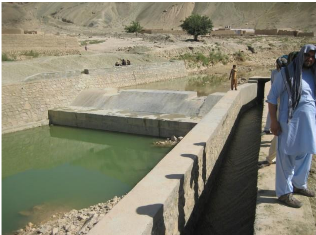
Figure 2: Weir+ Intake Built by Communities Contracted by MRRD under the Community-Based Irrigation Rehabilitation and Development Project
