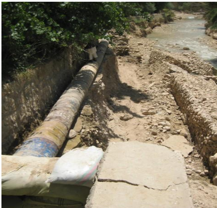
Figure 3: Destroyed Canal, Temporarily Repaired on Sarbagh River
