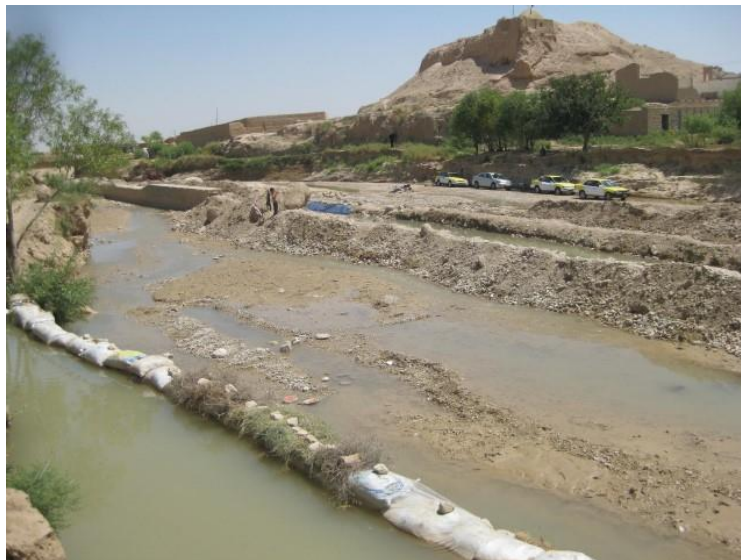
Damage to diversion and retaining wall, and sandbag canal repair Khulm, Balkh province.
